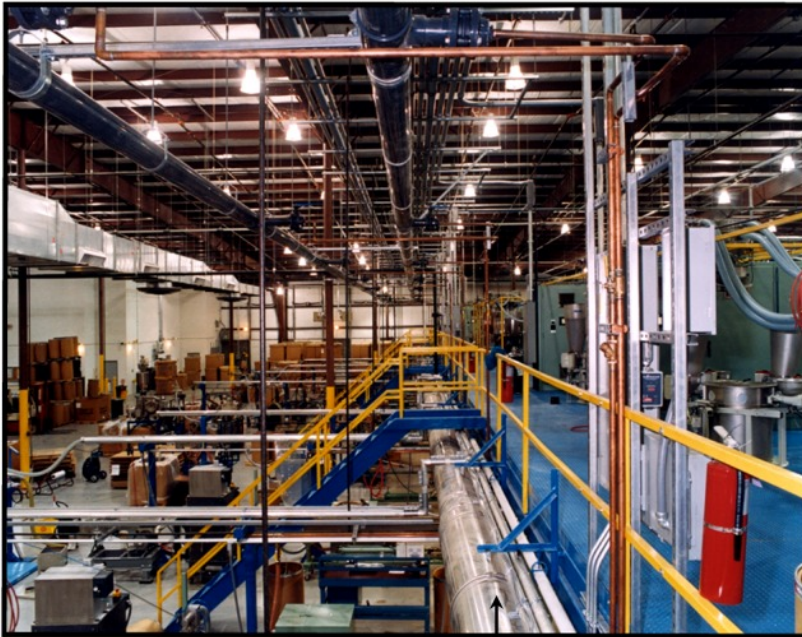
Fume Exhaust System with Scubbers
