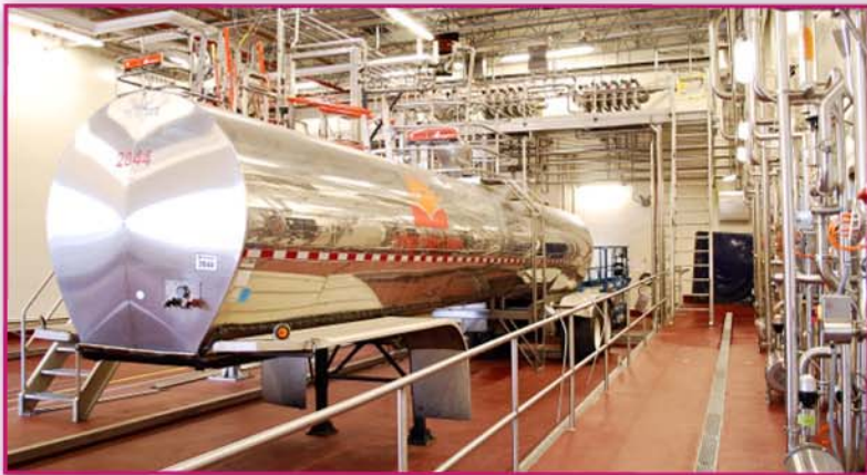
Tanker receiving bay
