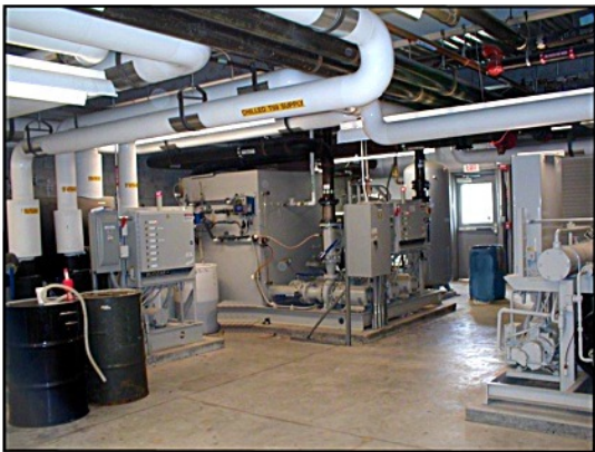
< Mechanical room in manufacturing building which houses the nitrogen generator, nitrogen storage tanks, feed air compressor, dryer for the nitrogen generator, cooling tower and tanks, chiller units and water heaters.
